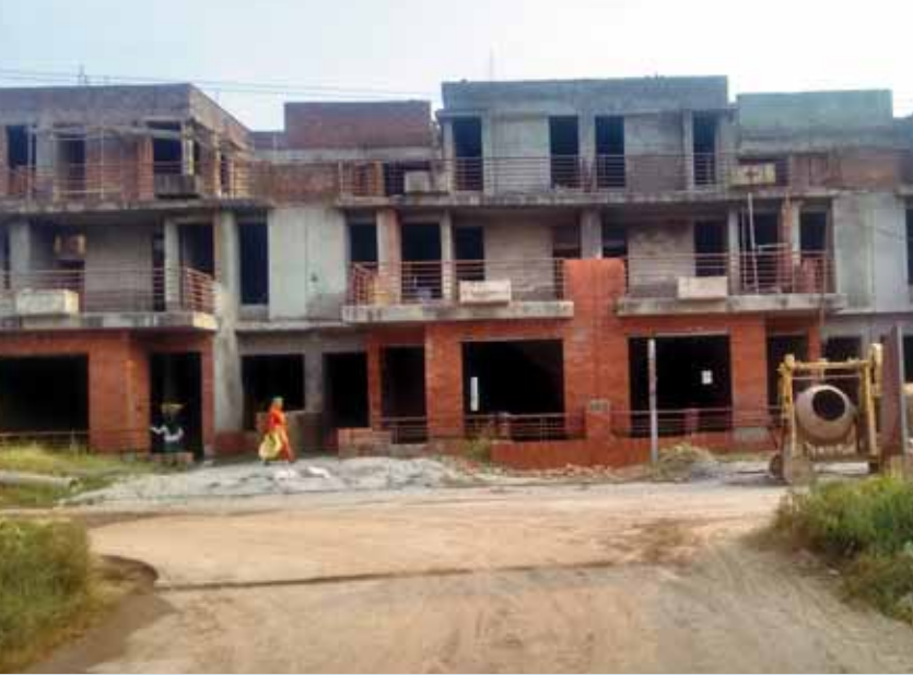
Internal Plaster & External Plaster work in progress in the row of 192 sq. yd. villas
